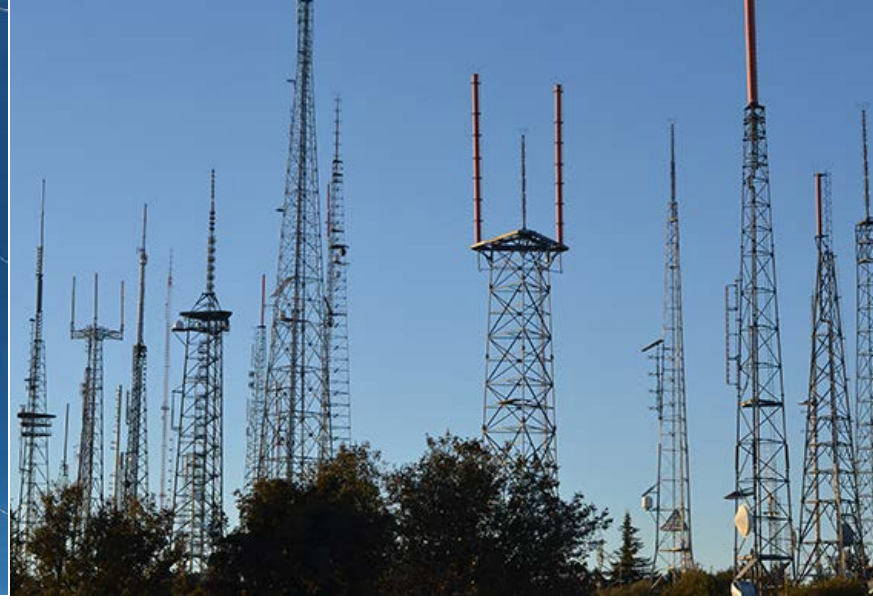
Congested mountain top site or building supporting multiple towers and multiple stations
